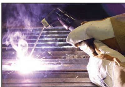
6) Hold the electrode slightly above the work piece to maintain the arc while travelling at an even speed to create an even weld deposition.
